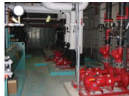
Water to water heat pump system
