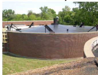
Covered tank / with Flare
